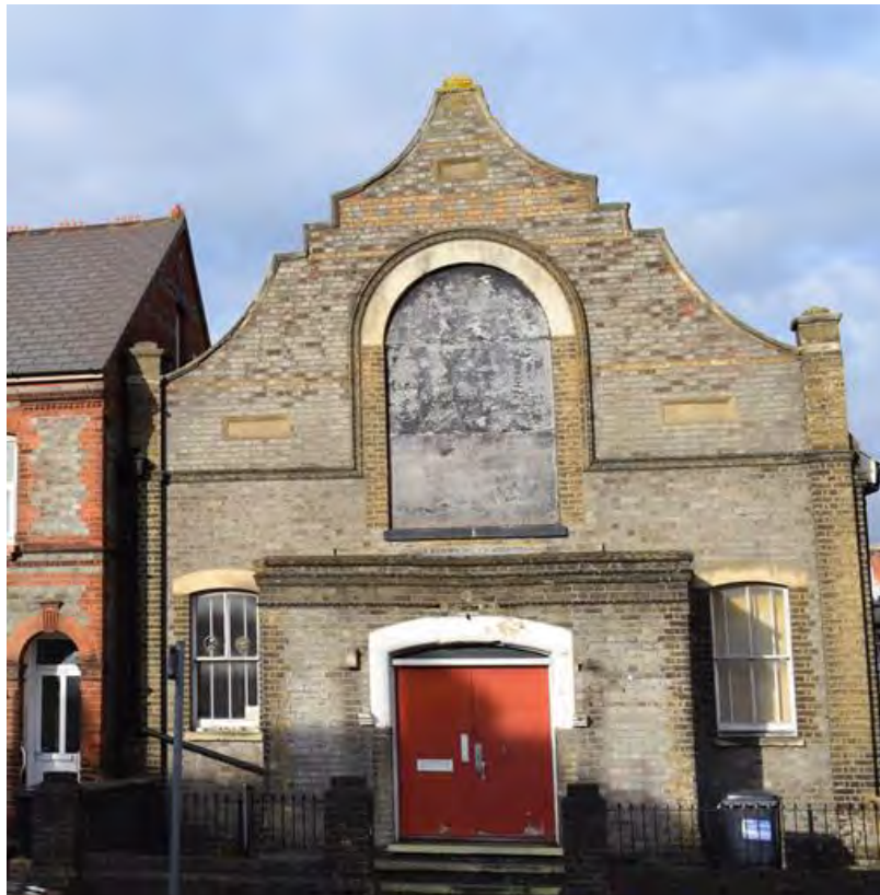
Figure 6.2.13 Bridge Hall, originally built for the Reading Open Brethren Group, in poor repair (David Neale)
