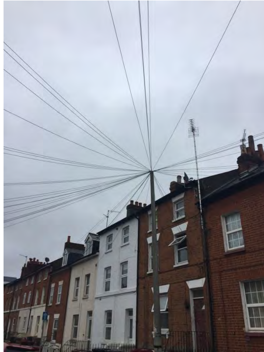
Figure 5.5.2 Overhead wires on a street with numerous HMOs (Karen Rowland)
